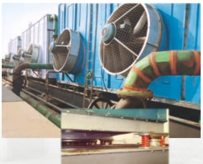
Roof Top Chiller installed on Spring Damper System
