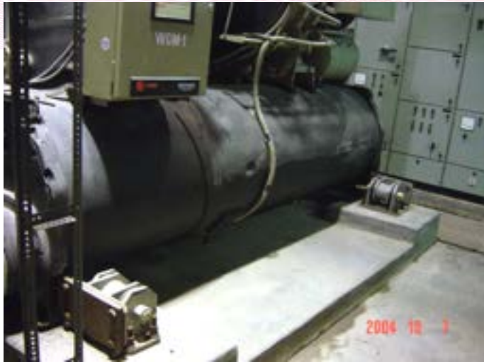
Seismic Snubbers protect HVAC equipments against Earthquakes
