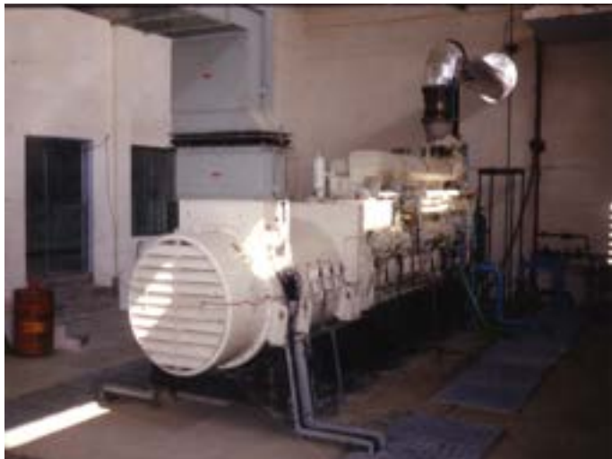
Base load Gen Set installed on Mountings without foundation
