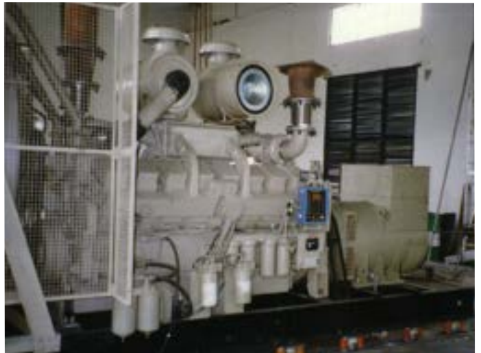
Diesel Gen Set on Spring Damper with over 95% Vibration Isolation
