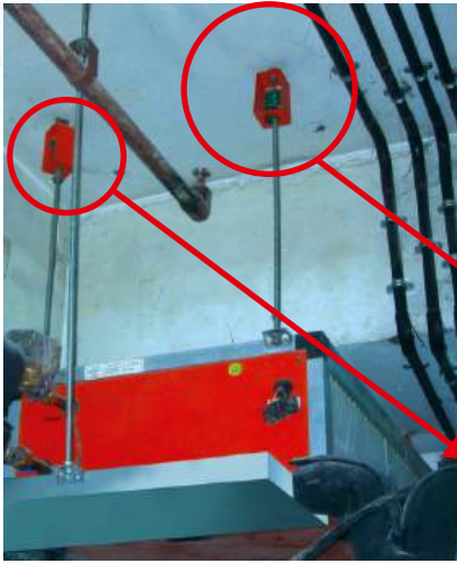
Fan Coil Unit suspended from ceiling using Spring Hangers
